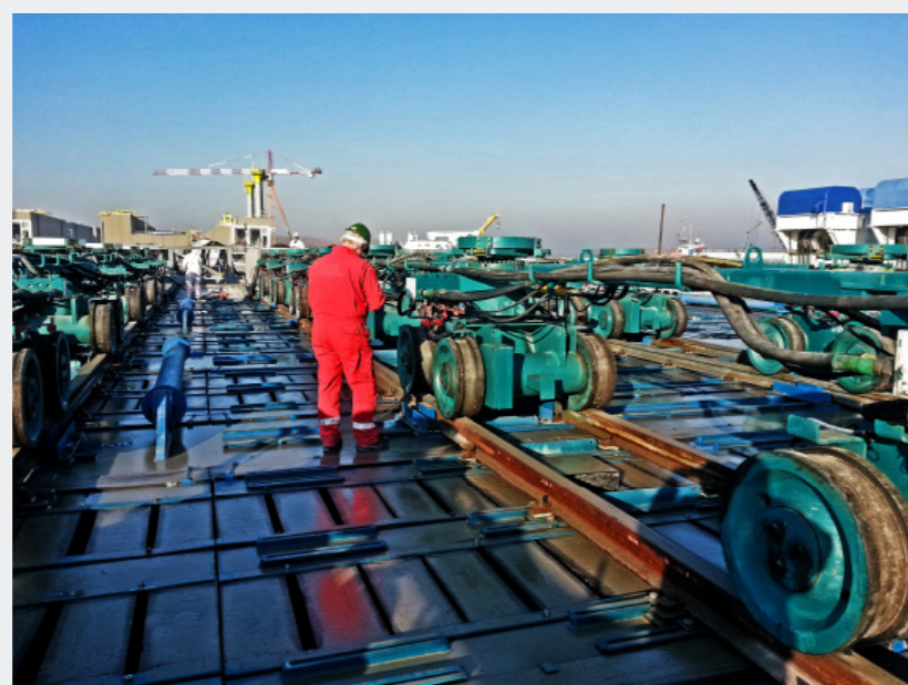
Inspections of Syncrolift equipment
